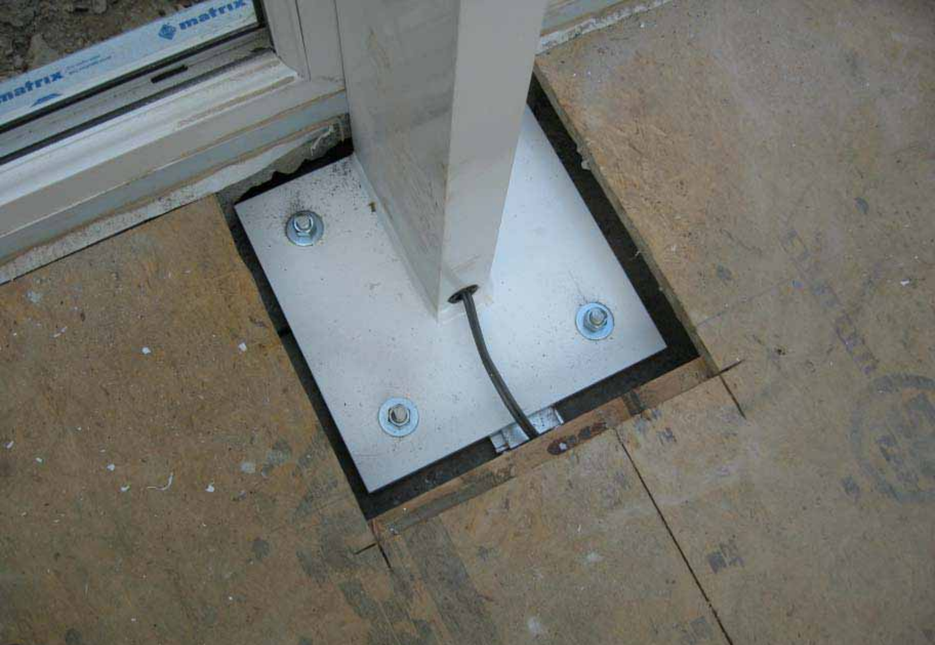
Picture Shows: Portal Frame Leg secured with Anchor Bolts to Concrete Piers
