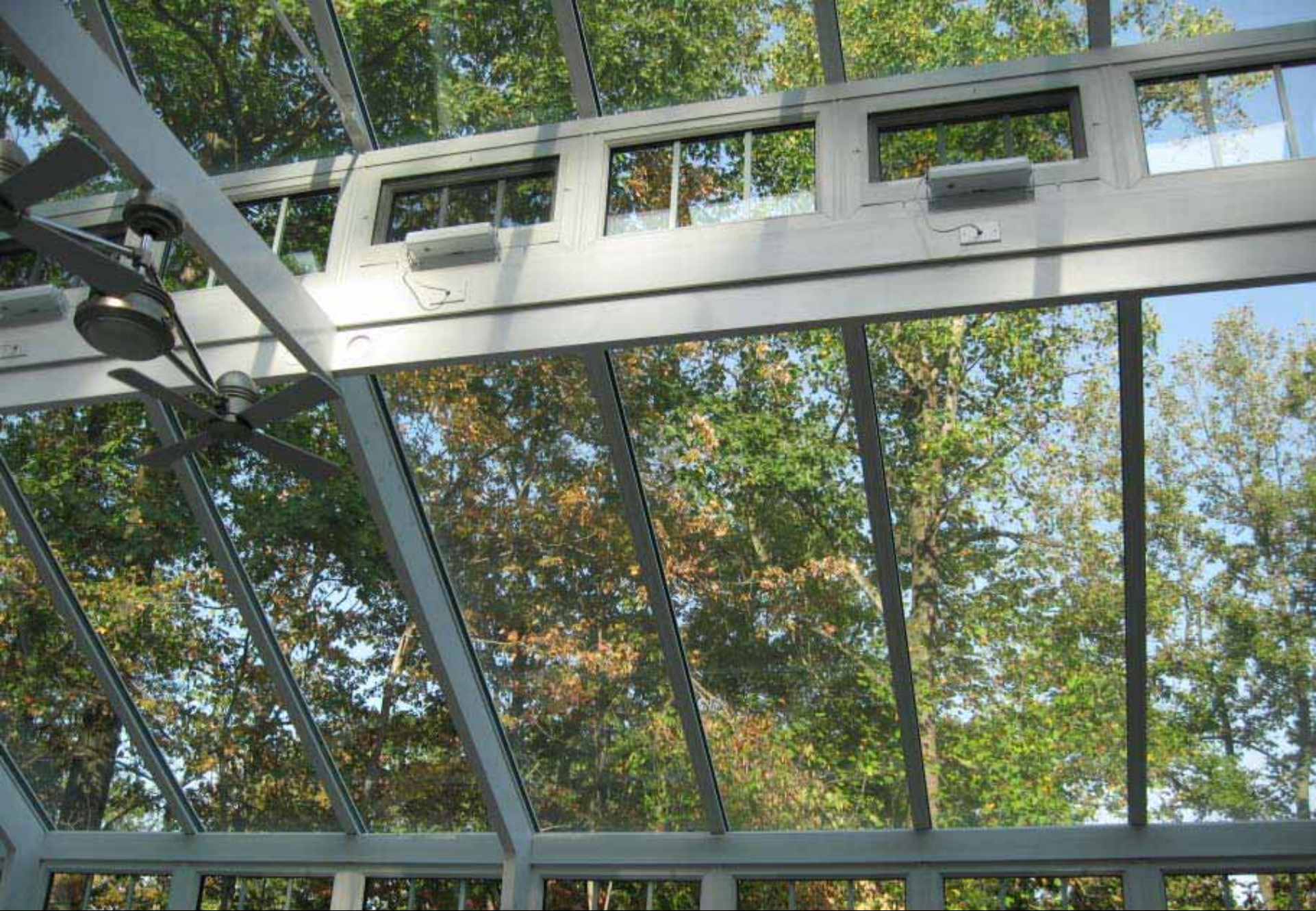
Additional View of Fan Installation and Motorized Lantern Vents
